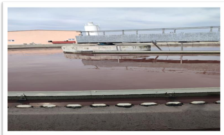
Slika 3. Ulaz obojene otpadne vode Figure 3. Inflow of colored wastewater
